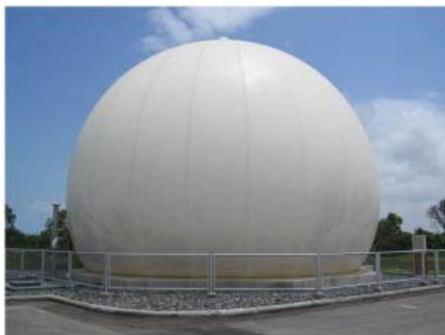
Rayong Municipality biogas storage tank
